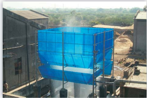
LTMCS installed on existing Cooling Tower pit
