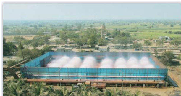
Largest LTMCS in operation, 4000 M 3 /Hr
